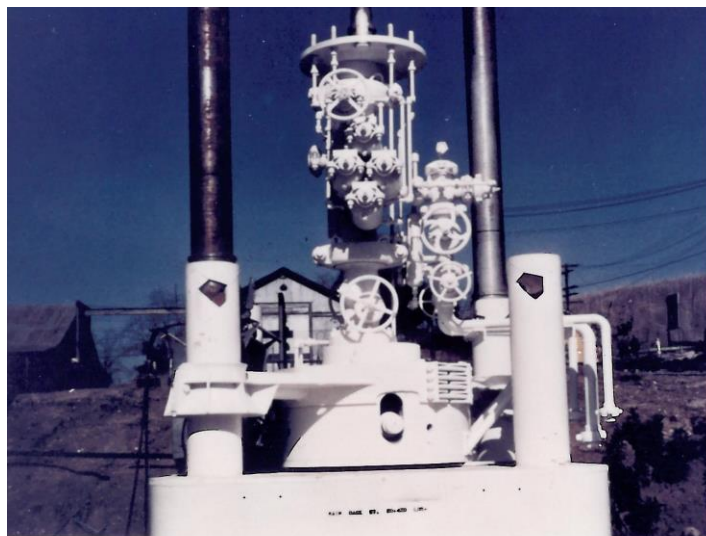
Caliente State #2 wellhead, circa 1964
